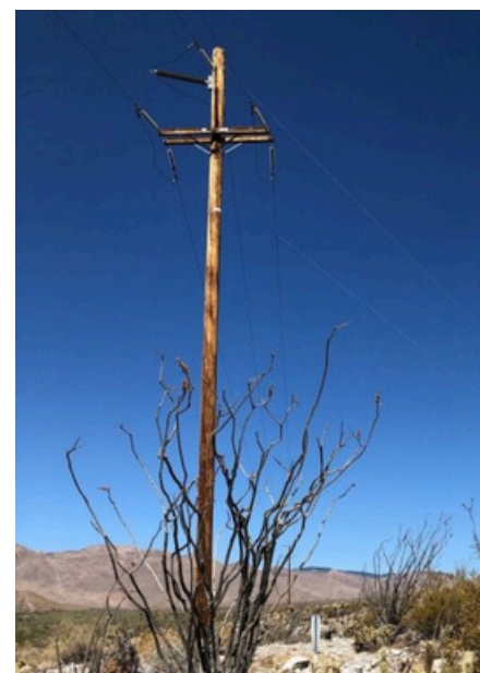
Existing Power lines
